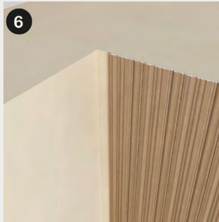
Measure the remaining space between the penultimate panel and the inner corner, considering the joints.
