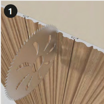
The damaged panel should be cut in two places as shown in the figure.
